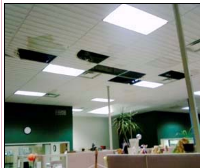
Ceiling tiles missing where rains poured in, soaking Colorado Springs field office.
